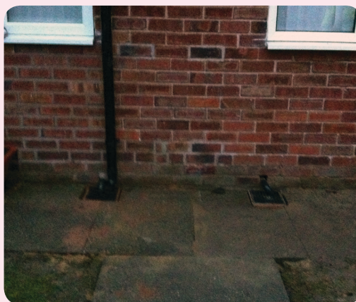
After excavation and partial reinstatement to ensure elderly residents could still access property safely.
