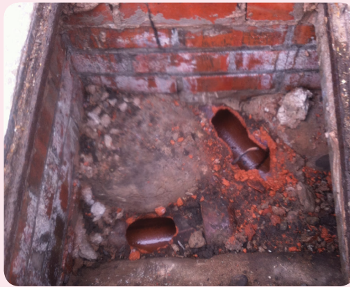
Existing manhole chamber in need of renovation
