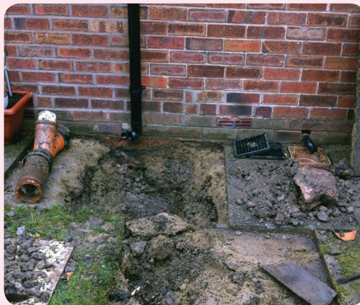
Excavation to remove poorly installed existing patch that was causing residents toilets to block.
