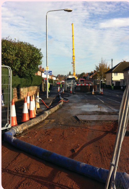
Overpumping Pipes and a pumping system controlled water flows during the lining process.
