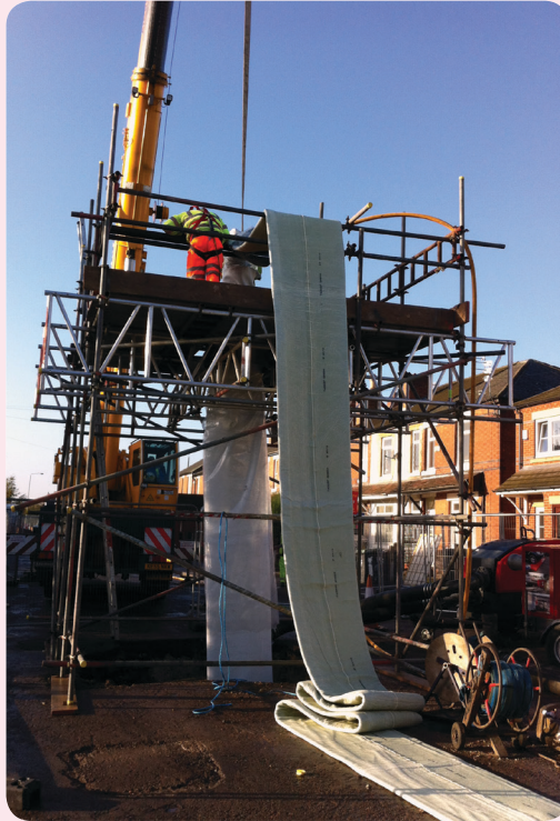
Liner installation Proximity of houses shows how sensitivity to disruption was paramount throughout this project.
